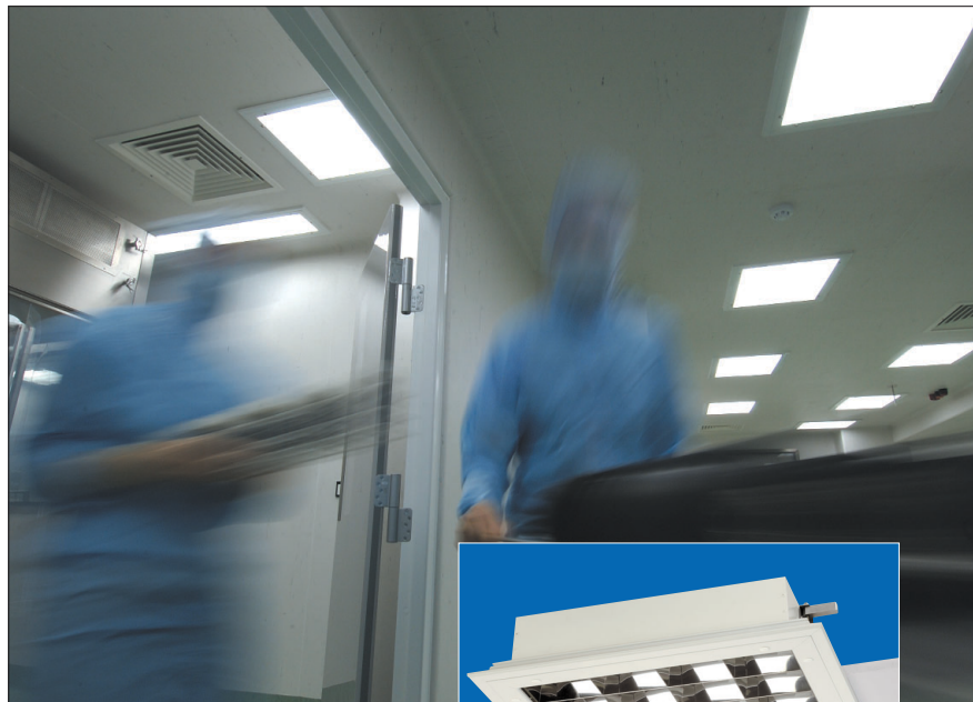
DTFN in an FS200D class 10000 clean room with non modular ceiling.
