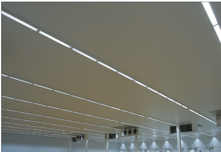
DTBY on a solid ceiling in a food process plant
