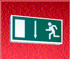
EMX EMERGENCY LIGHTING PAGE 251
